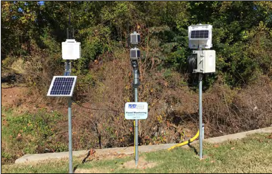
Low Cost Flood Sensors
