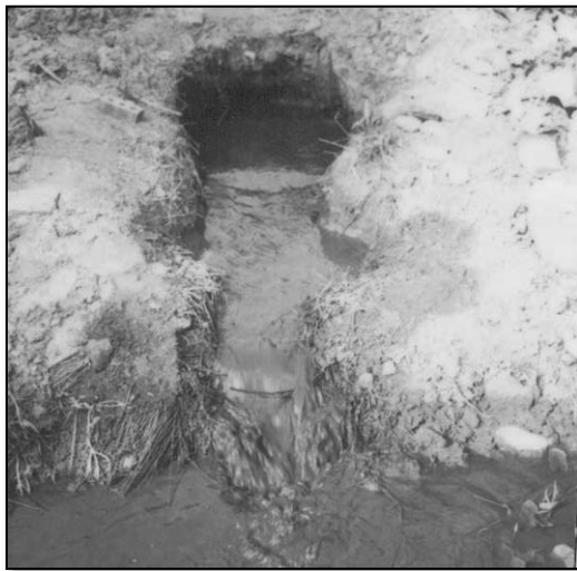
Sewer Line Bypasses Straight To Creeks
