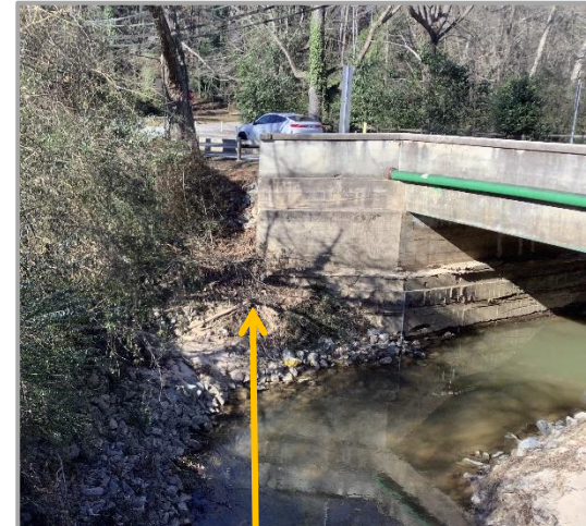
Historic scour issues and roadway runoff
