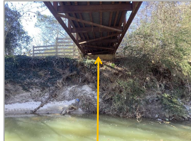
Bridge foundation scour
