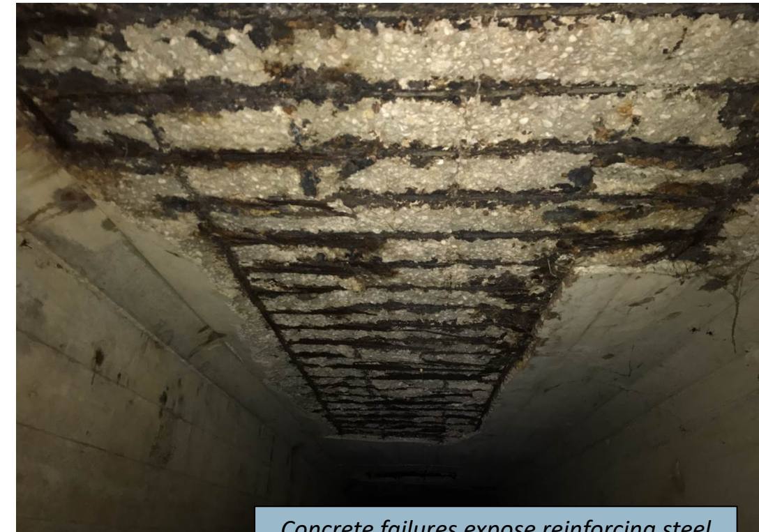
Concrete failures expose reinforcing steel in a box culvert, causing a serious concern
