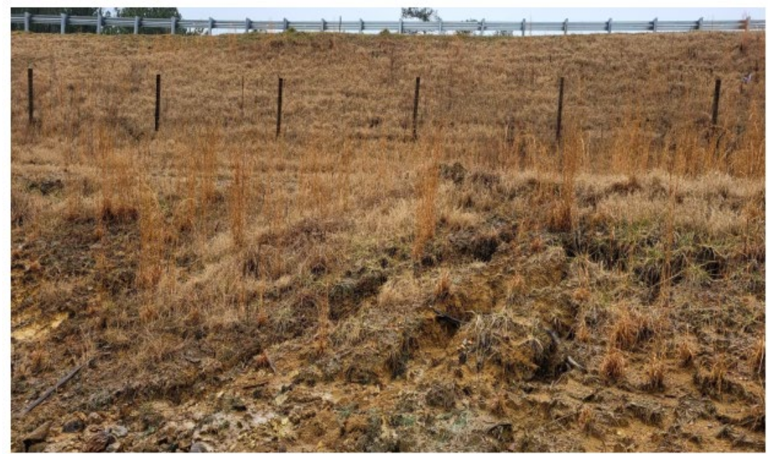
Interior slopes have experienced excessive rill erosion
