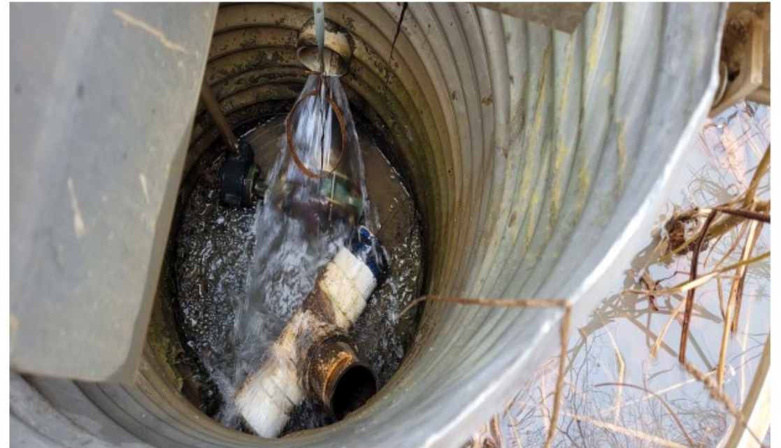
The drawdown upturn device needs repair
