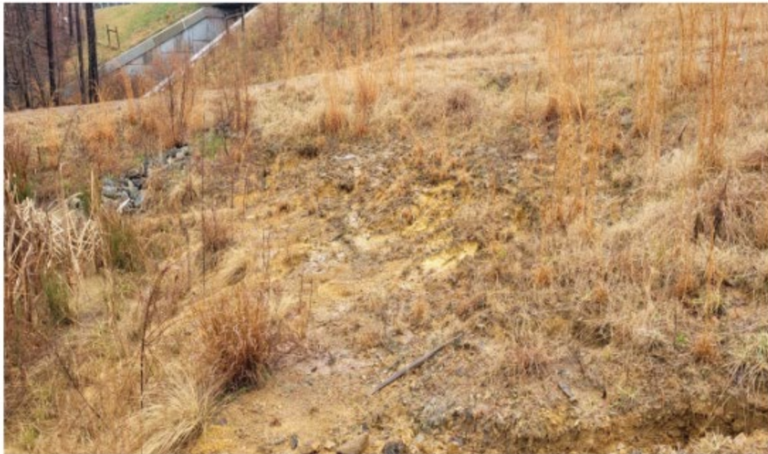
Interior slopes have experienced excessive rill erosion
