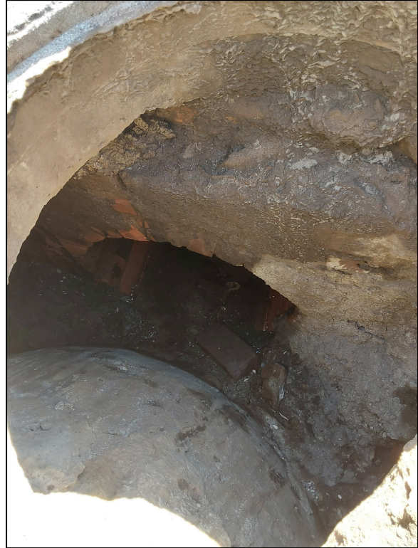
Ageing brick lined conveyance structure located in Craven Street and Charles Street intersection.
