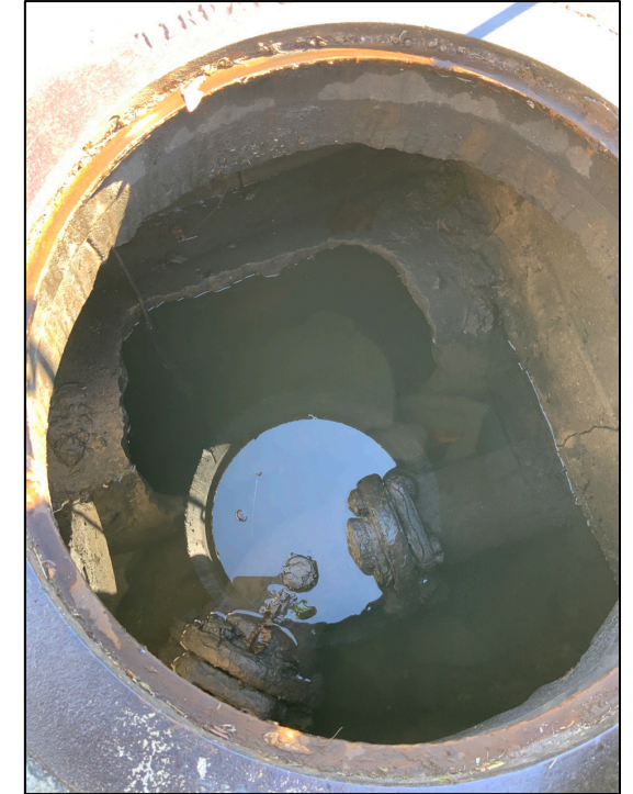
Manhole structure containing broken stormwater pipe and exposed water line near Port Republic Street and Carteret Street intersection.
