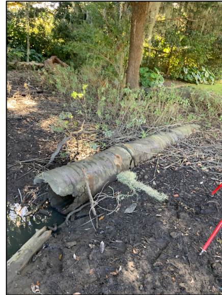
Degrading outfall pipe off East Street between Craven Street and Port Republic Street.
