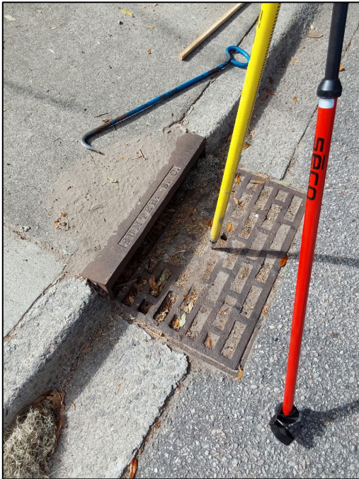
Silted type 1 grate inlet near Greene Street and West Street intersection.
